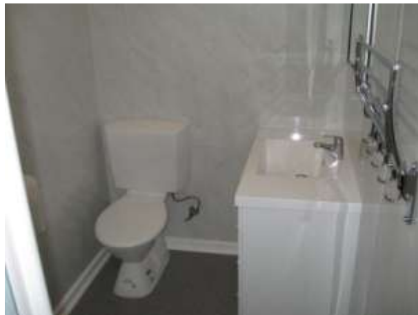
New hand basin and cupboard, floor covering, skirting boards, cistern, toilet and towel rack
